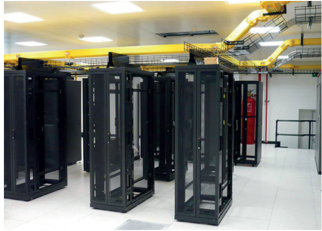
Typical installation of overhead copper and fibre management system with customised brackets to the top of the cabinets
